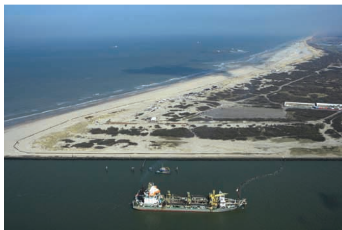
Beach nourishment for a dune compensation project on the Delfland Coast, the Netherlands. Sand is pumped to site through a pipeline crossing the 'Van Dishoorn triangle', a land reclamation near Port of Rotterdam.
