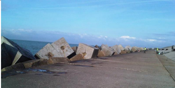
Figure 1. Concrete blocks containing contaminated sediments on the 'Digue des Huttes' in Dunkirk (Septembre 2013).
