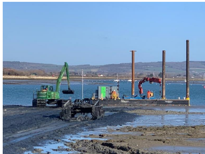
Drag box being trialed at West Itchenor in February 2023 (c) Land & Water Services Ltd
