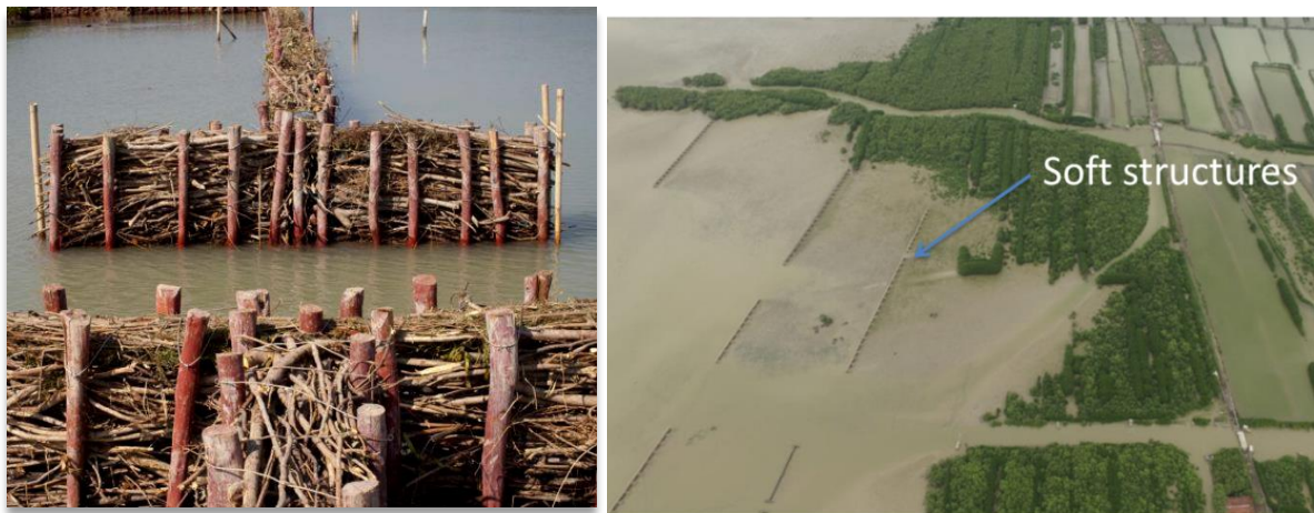
Figure 1. Soft permeable structure. Close up (left) and implemented in the field (right)
