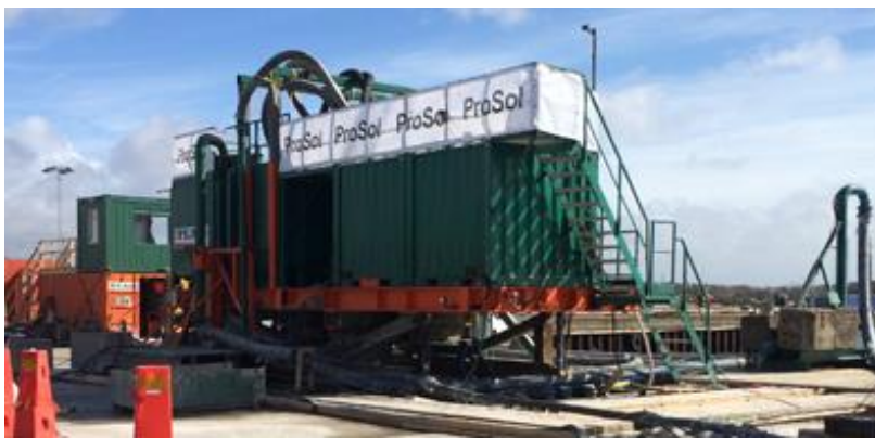
Figure 2. Binder/sediment mixing plant provided by PEAB
