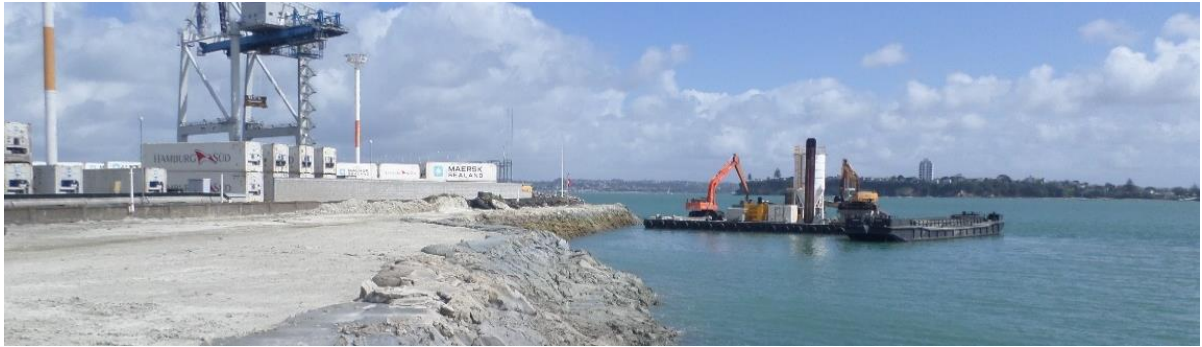
Figure 1. Image of the Heron Construction Co Ltd's Mesenge pugmill barge processing dredged material from a hopper barge and placing at the Port of Auckland reclamation.
