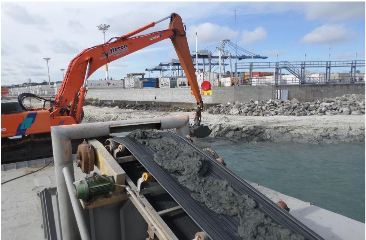
Figure 2. Mesenge pugmill barge's EX700 longreach excavator placing mudcrete at the Port of Auckland reclamation.
