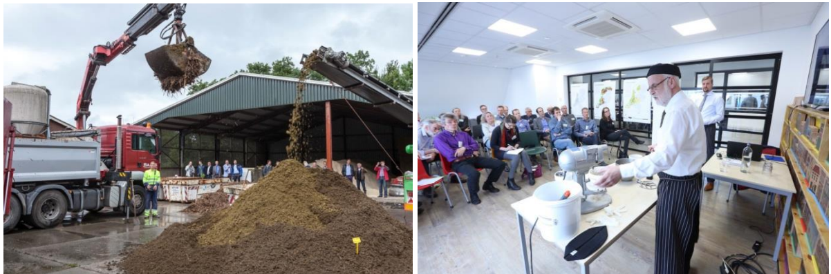
Figure 3. Mixing of Topsurf during demonstration on-site (left); Workshop on Topsurf during congress on land subsidence (right)
