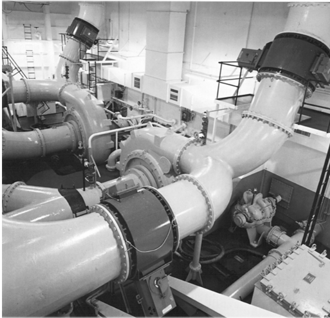
Figure 2-30 Pump room with 2 pumps
