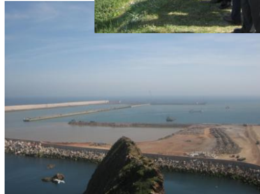
Dredgers pumping sand into the reclamation area at the Port of in Gijón.
